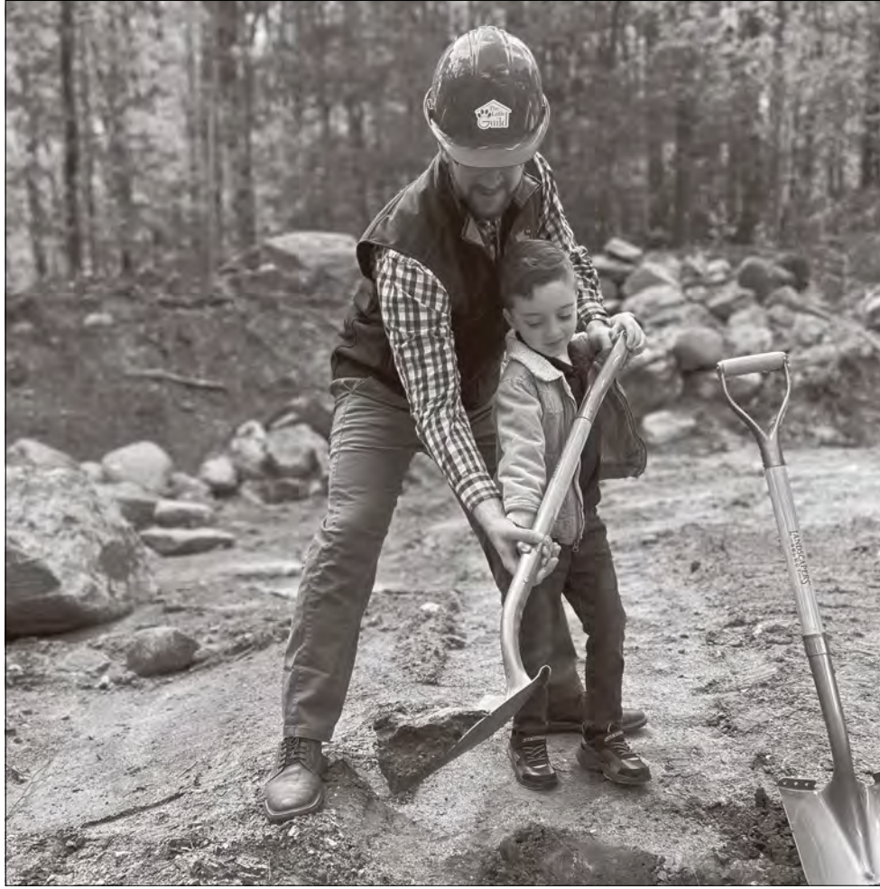
Architect Christopher Nardi and his son Everett break ground for the new home of The Little Guild in West Cornwall.
