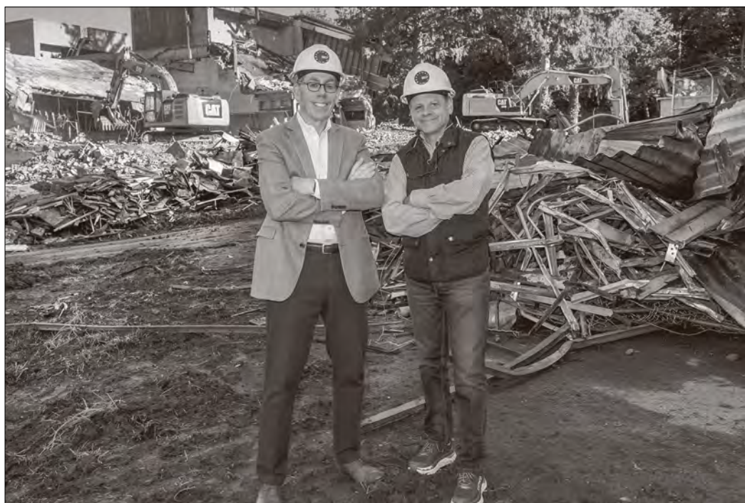
Left, Millbrook Community Partnership (MCP) Treasurer George Whalen and MCP President Oakleigh Thorne stood at the site of the demolition taking place at the former Bennett College campus. Plans for a 32-acre park are underway.
