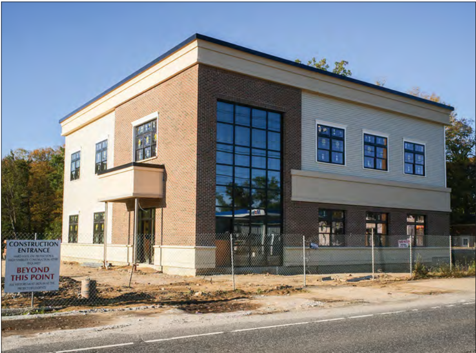
The Community Health and Wellness Center on Route 44 in North Canaan.
